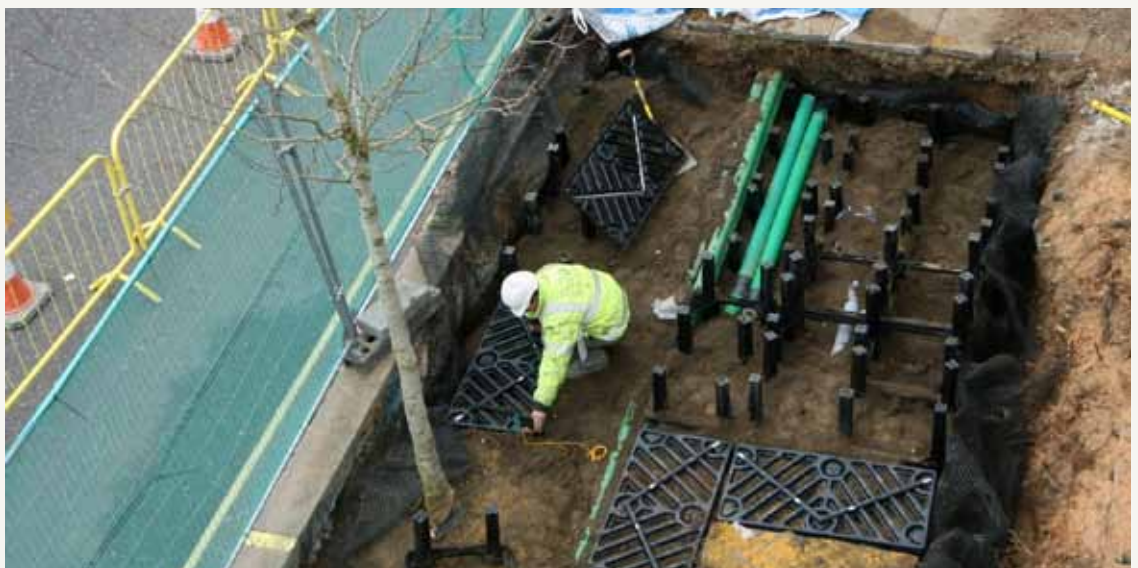
Installation of the 'Sylva Cell' modular cell system ensuring news street trees planted in front of the new RAF Bomber Command Memorial in London will grow big. © Jeremy Barrell
